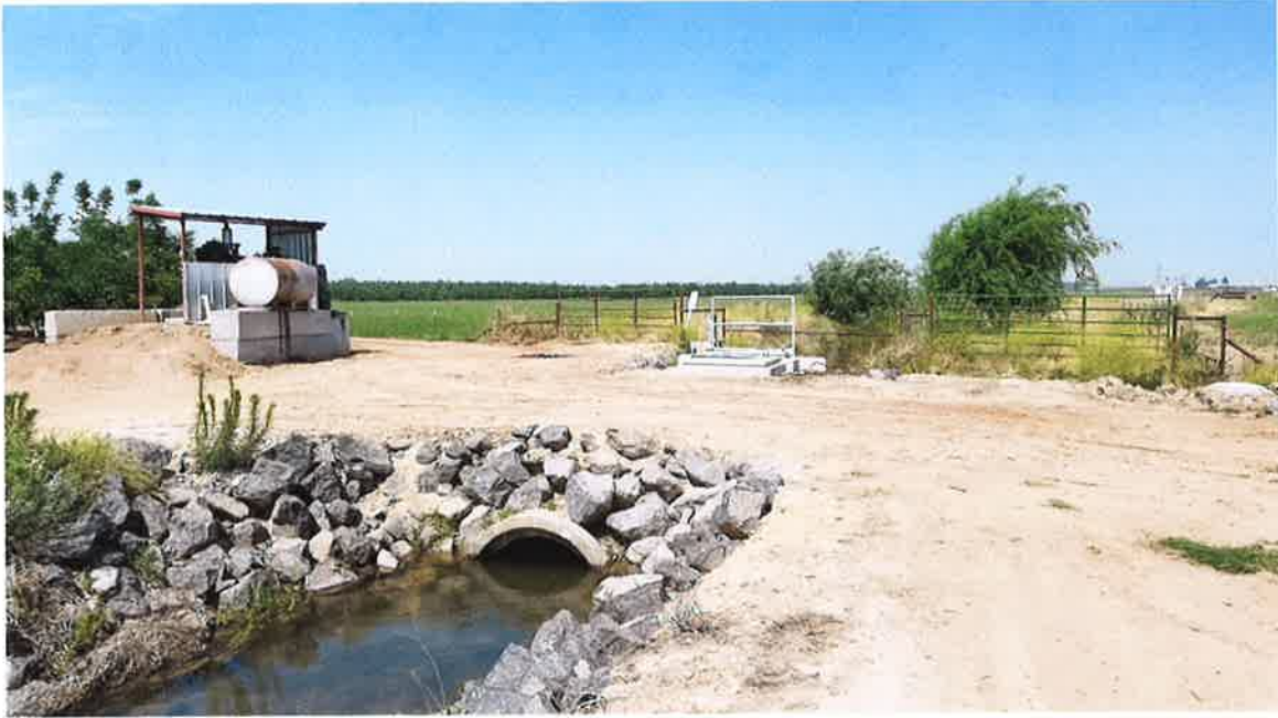
Looking east immediately downstream of private pump station for APN: 014-005-003 and backup structure for existing delivery point.
