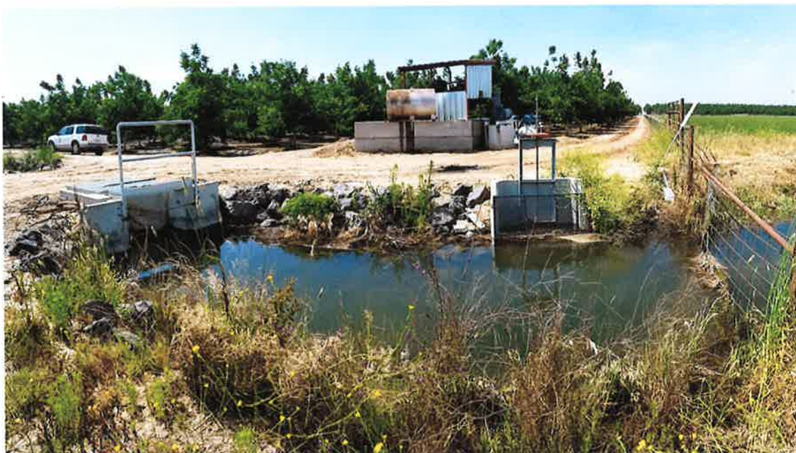
Looking north near the shared property line of APNs: 014-005-003 and 014-00-008. Private pump system, current delivery point, and backup structure under operating conditions for APN: 014-005-003.
