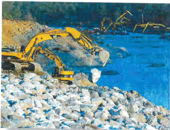
RSP - Oroville Dam Spillway Emergency Response
